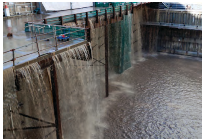
Figure 5: Flooding of the Vision Tower Brisbane construction site in 2011. (Source: Brisbane Development)
