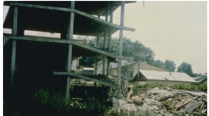
Figure 1: A building under construction following severe earthquake damage. (Source: NOAA/NGDC, M. Mehrain, Dames and Moore)
